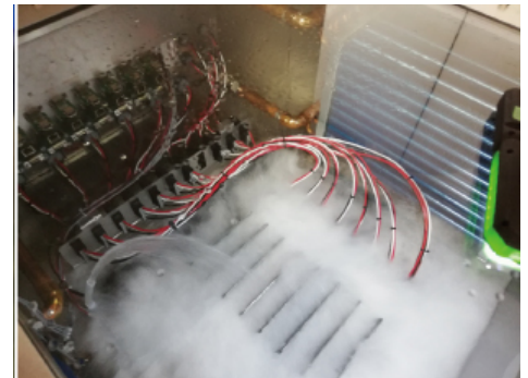
Servers and other IT equipment are submerged in a non-conducting dielectric fluid.
